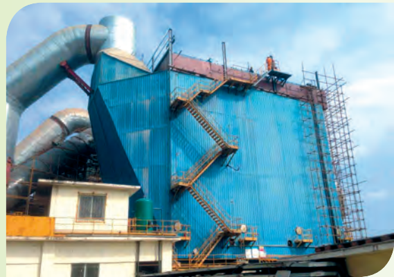
華潤水泥（田陽）有限公司1#窯頭除塵器改造 Transformation of dust collection system at 1# Kiln of China Resources Cement (Tianyang) Limited
