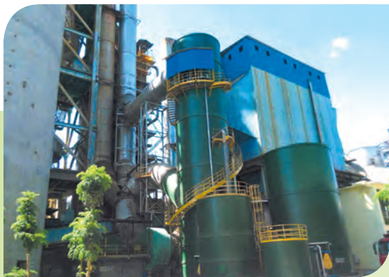
華潤水泥（陽春）有限公司脫硫系統 The desulphurization systems in China Resources Cement (Yangchun) Limited
